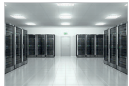
Fig.: Constant processes and highly sensitive applications such as data centres, are based on RCM monitoring.
